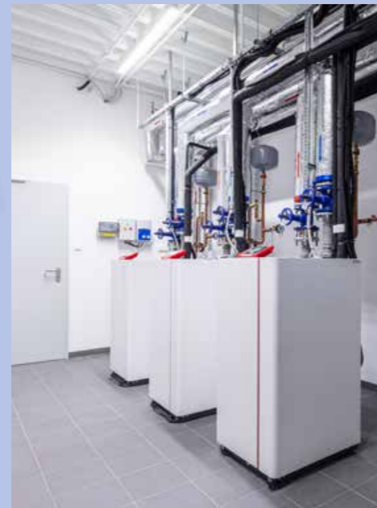
Heat pump room in modern commercial building.
